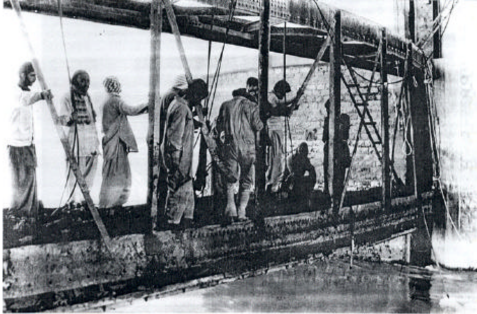
Fig. 6. The lower and upper bow-string girders each having its own horizontal braces and vertical braces connecting the two. Note that the horizontal braces of upper bow-string are in line of the lower one have folded and warped, and bow and string girders of lower one are almost touching each other, save for the crushed braces between them.
